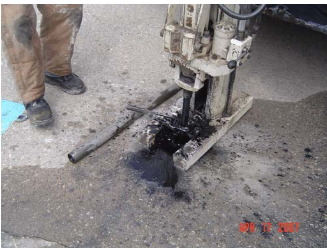
Photo#5 KSF-SB-05 Coal tar flowing out of drill rods
